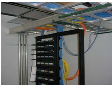
Voice & Data Network Infrastructure
